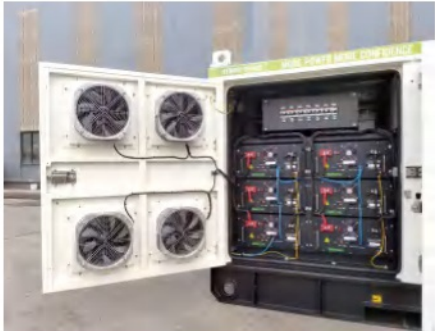
For Greener Power Solutions
